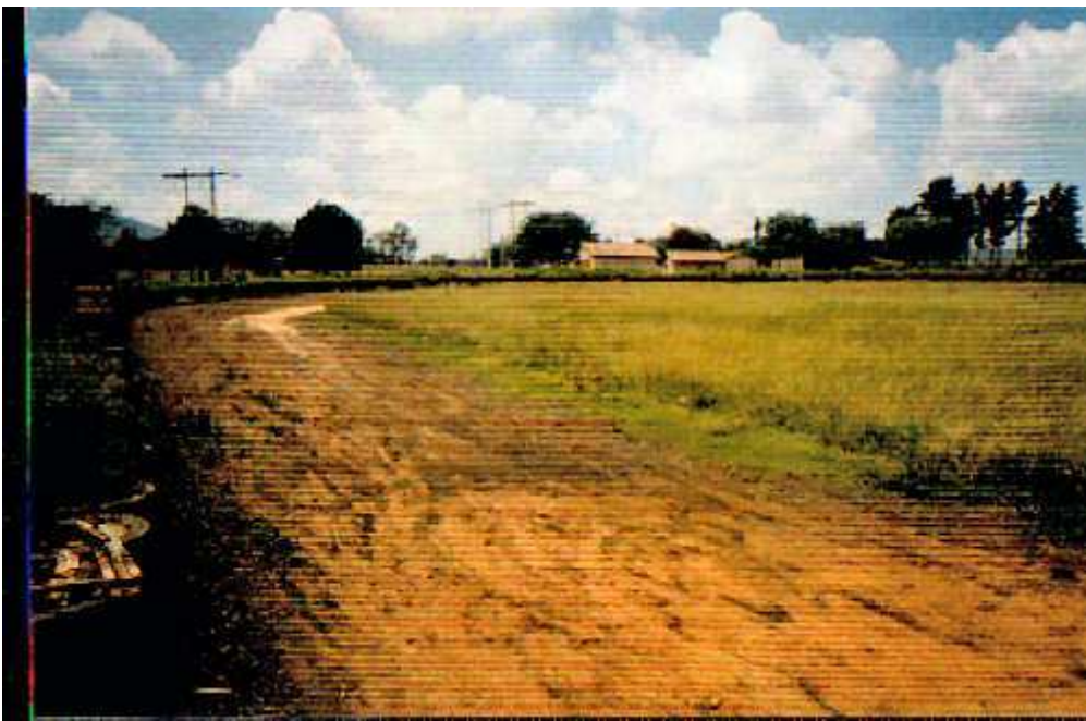
Marking out the track in the field - the first earth has been removed
